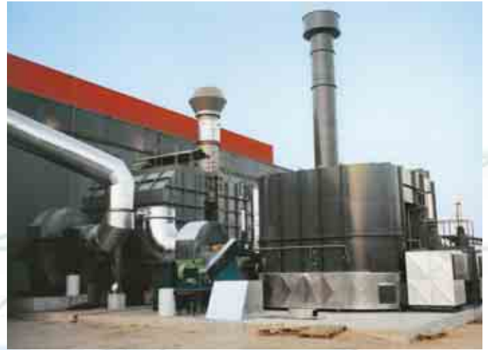
Superficial coils treatment • Twin regenerative oxidisers 45,000 Nm 3 /h installed in different period of times
