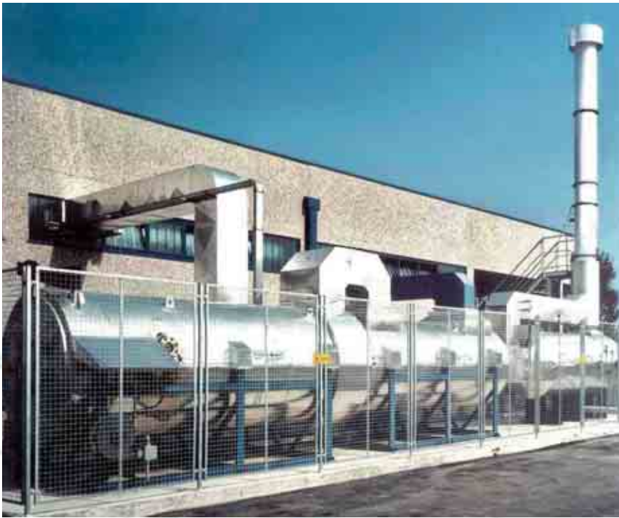
Flexible Packaging Printing Effluent gas • 18,000 Nm 3 /h • Thermal Fluid Heat Recovery
