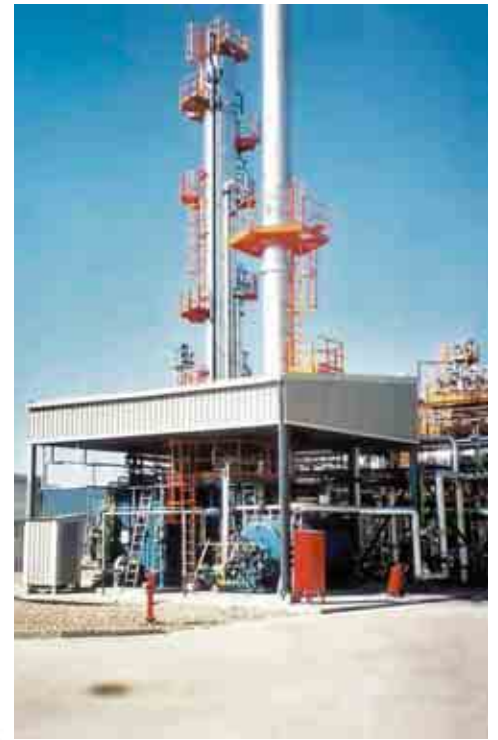
Petro-Chemical Plant Oxidiser with integrated thermal fluid heat recovery
